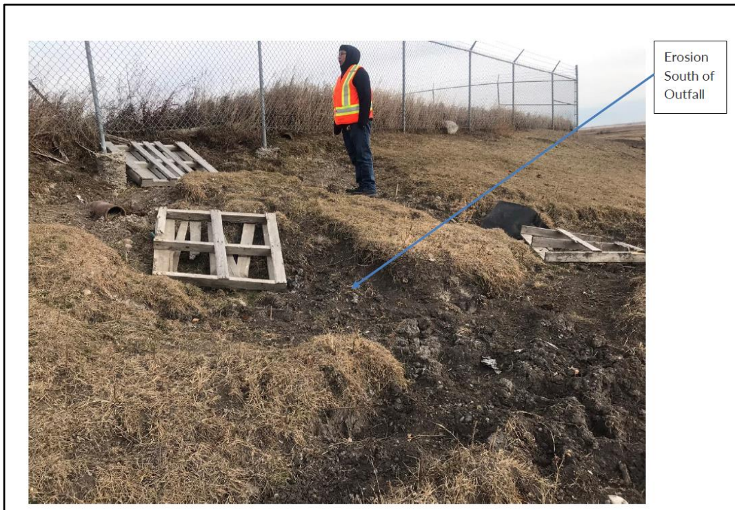
Erosion at outfall of Cell 4
